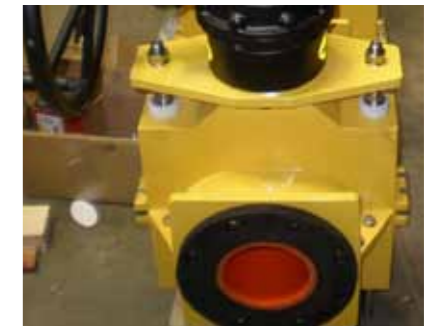
Lime Dosing Manual Pinch Valves
